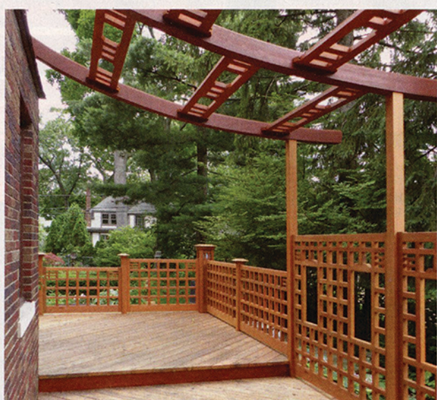
The curved cedar trusses (top) and grid-style panels (above center) were fabricated in the authors’ California shop, then shipped across the country to the jobsite in Michigan for installation (above).
