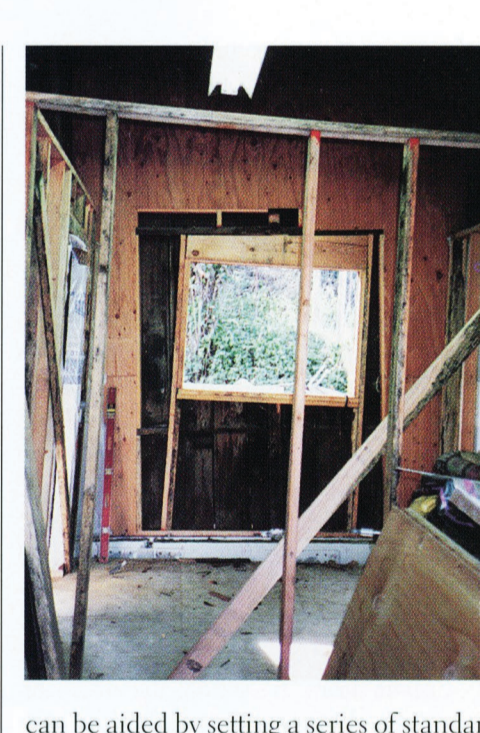
can be aided by setting a series of standard house jacks beneath the ridge board and connecting them with shoring timbers. Beginning with the center come-along and moving outward, the cables are tightened gradually in an even sequence that avoids too much stress in any one area. Take your time, putting just a half-turn a day on each device.
